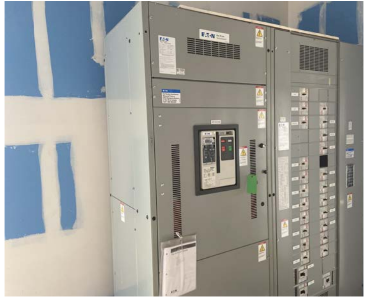
Electrical switchgear in IL
